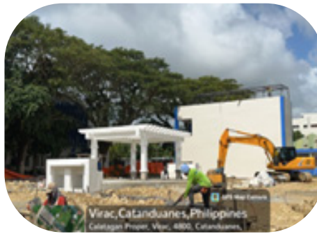
WATER CATCHMENT BASIN NEARING COMPLETION. To be used in recycling rainwater, the construction of a catchment basin at the back of the Catanduanes State University's administrative building is set to be completed this year, among the projects included in the approved Land Use Development plan.
