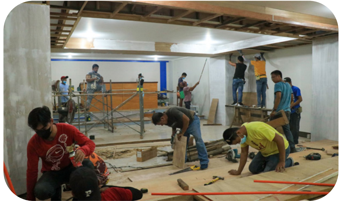
ON THE GRIND. Workers are on the move of crafting and grinding the moot court of Catanduanes State University, one of the requirements to offer Juris Doctor program under the College of Law.
