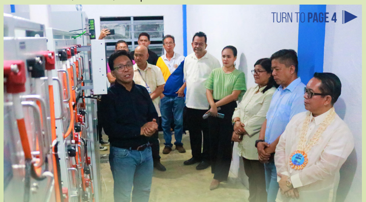
LIGHTS ON. General Manager Rodolfo M. Romero of contractor Gentromech Co. shares the unique features of the CatSU Solar Microgrid (Hybrid Solar Farm) during its launching.
