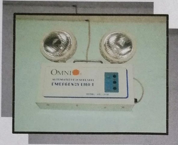
Emergency light is mounted just above the safety procedures bulletin and is located at the right side of the room.
