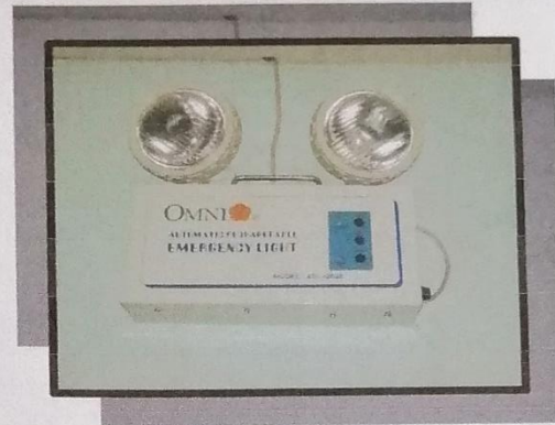
Emergency light is mounted just above the safety procedures bulletin and is located at the right side of the room.
