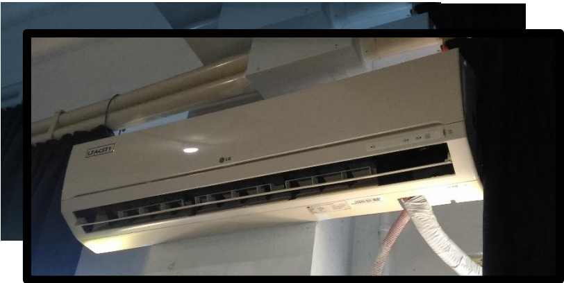
An airconditioning unit is used as a ventilation for the laboratory room
