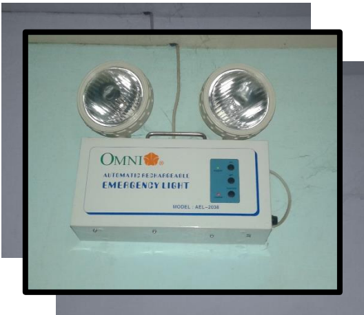
Emergency light is mounted just above the safety procedures bulletin and is located at the right side of the room.
