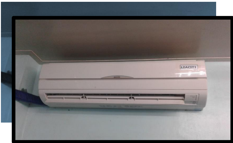
(above image) two airconditioning units are placed on computer lab 2 mounted on opposite walls of the wall.
