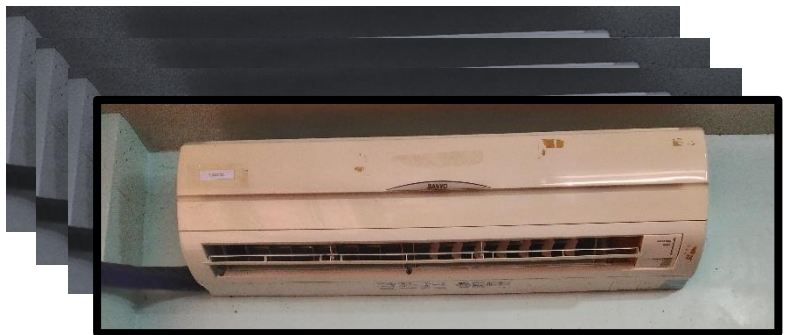
Two airconditioning units are mounted at adjacent sides of the room
