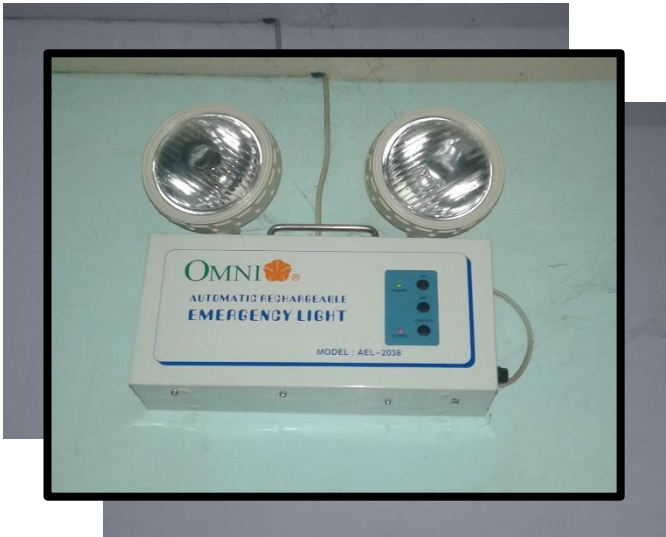
Emergency light is mounted just above the safety procedures bulletin and is located at the right side of the room.
