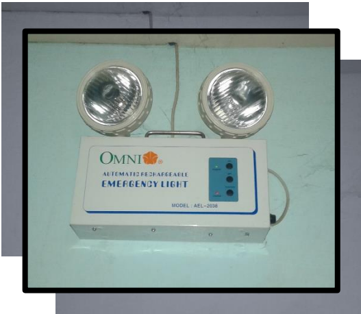
Emergency light is mounted just above the safety procedures bulletin and is located at the right side of the room.
