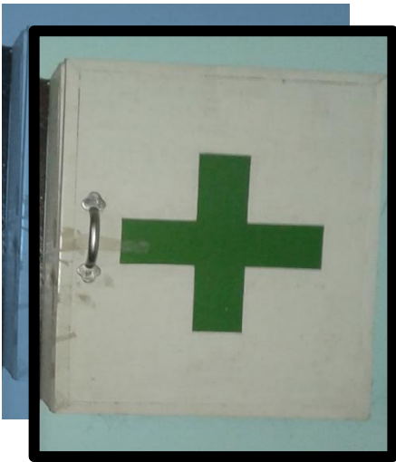
First-aid kit is mounted on the wall just beside precautionary measures bulletin and they are located at the left side of the door
