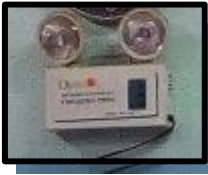
Emergency light is mounted just above the safety procedures bulletin and is located at the right side of the room.
