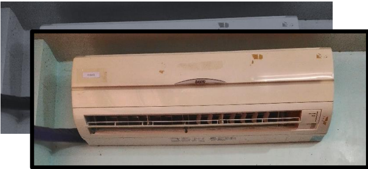
An airconditioning unit is used as a ventilation for the laboratory room
